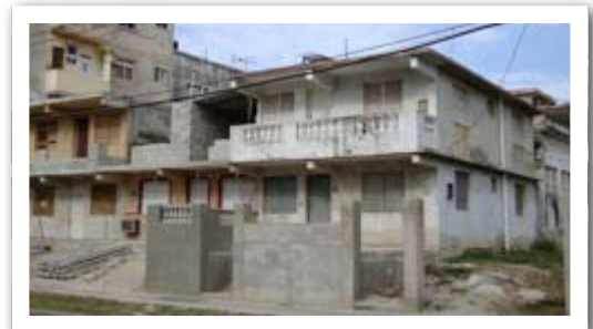
I watched the two corner houses being built over more than 6 years. They have been occupied for the past 2 years as the building continues.
